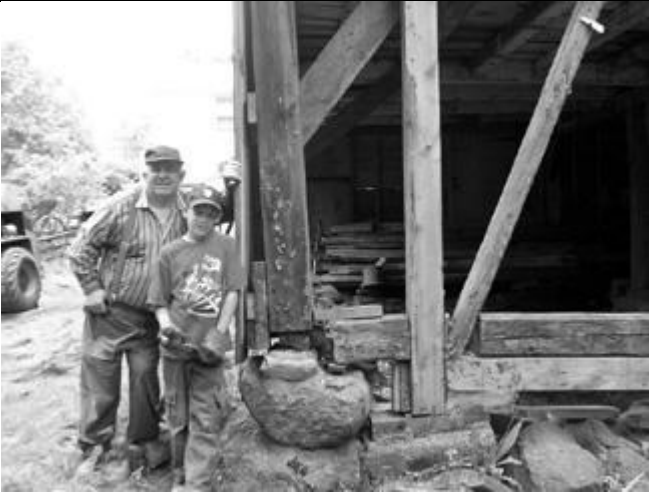
Jim Gaskell's grandson, Peter Pekkala, with Richard Crane holding up rear side of the barn during replacement of beams in basement
