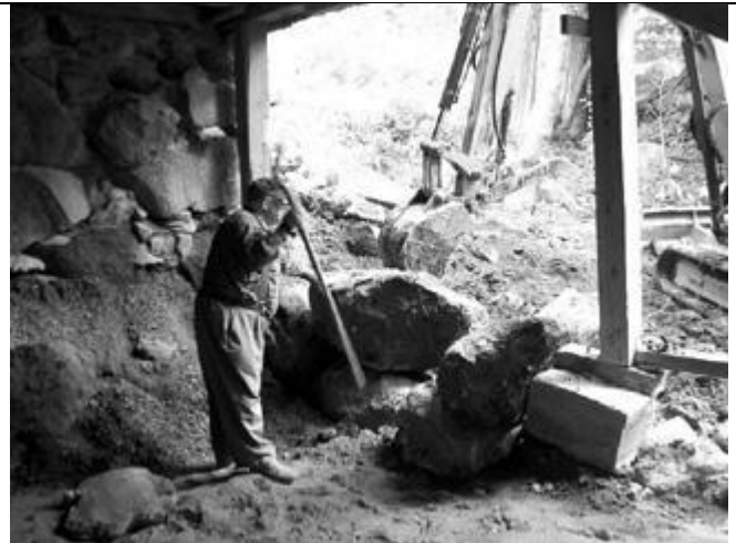
Richard Crane directing excavation operations from a safe place in the basement
