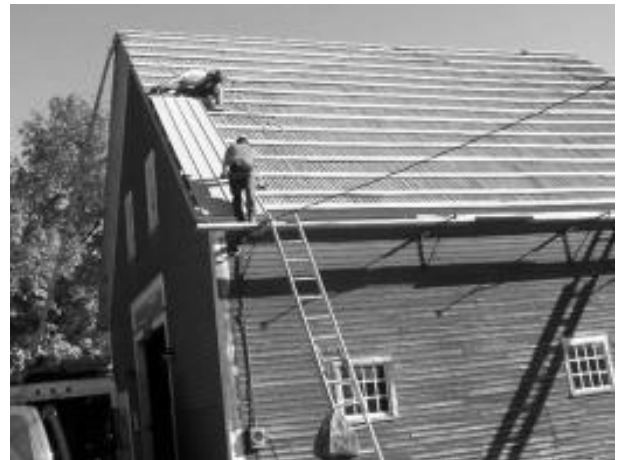
Contractor workmen installing the first section of new roof - Note safety ropes
