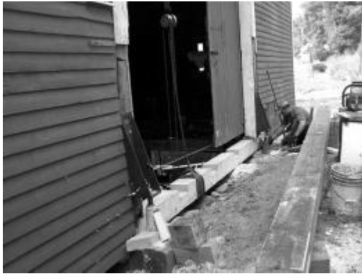
Contractor laying new sill beam across front entrance (beam prepared by Phil Barker with his portable sawmill)
