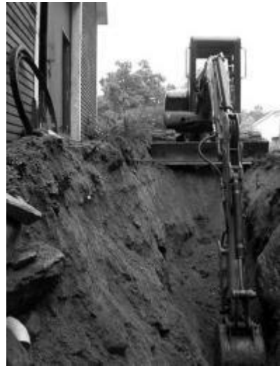
Phil Barker operating excavator to dig new deep drainage ditch across front of barn
